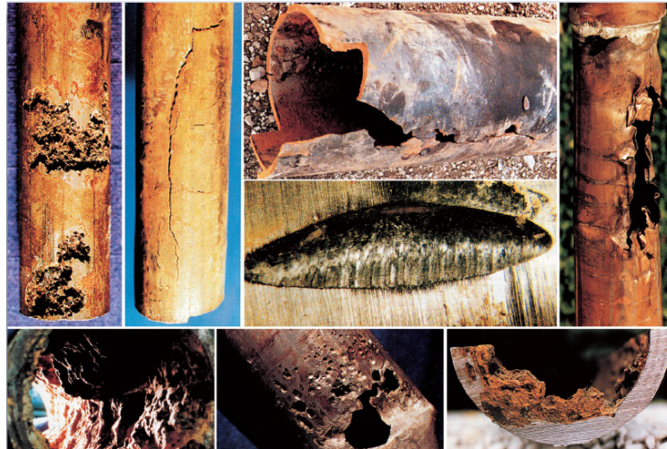
La corrosion - © Suez
